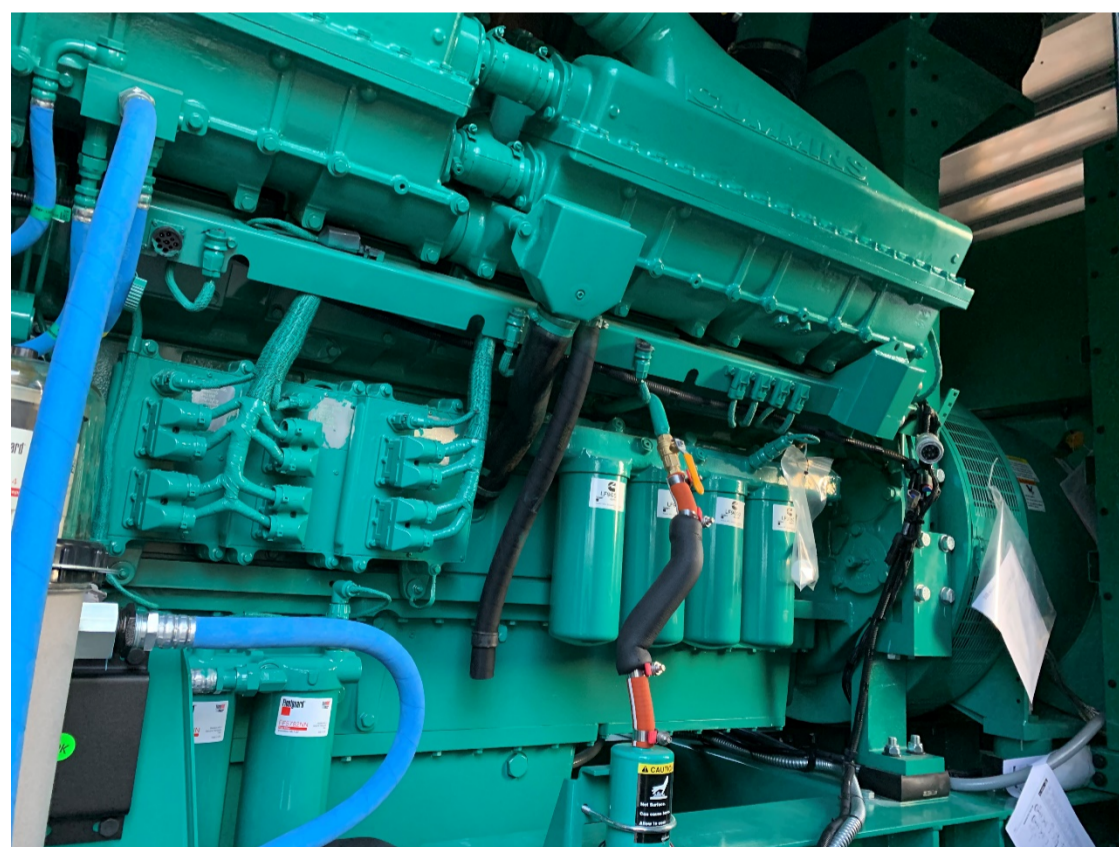
Figure 12: UCI Blackstart Generator
