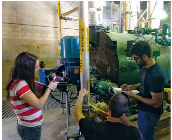
UCICL students (Jamie Ibrahim, Nathan Kirksey and Dimas Avila) document dimensions of the fuel gas delivery system for "Boiler #2" at the Chiquita Water Reclamation Facility.
